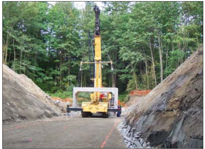
A crane lowers one of the first sections of the culvert into place.
