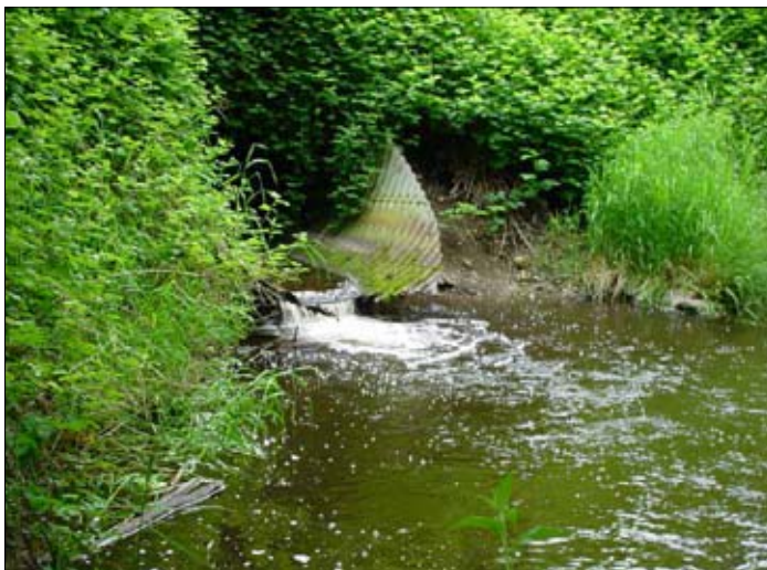
The broken ends of an old steel culvert flipped up when water was running high, blocking passage for fish trying to swim upstream. The broken culvert also was an indication that water could be seeping in around the pipe, jeopardizing the road above.
