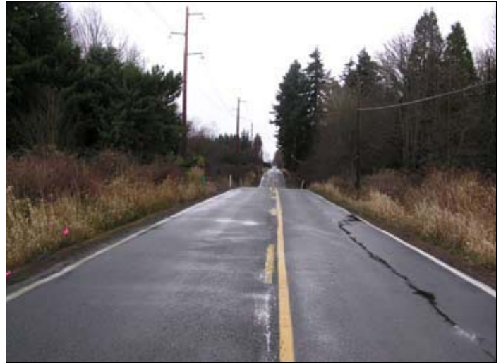
WSDOT took the opportunity to flatten a dip in State Route 548 in Whatcom County while they were replacing a culvert.
