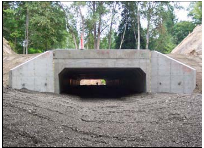
Crews laid streambed gravel across the base of the new culvert creating a seamless transition with the natural streambed.
