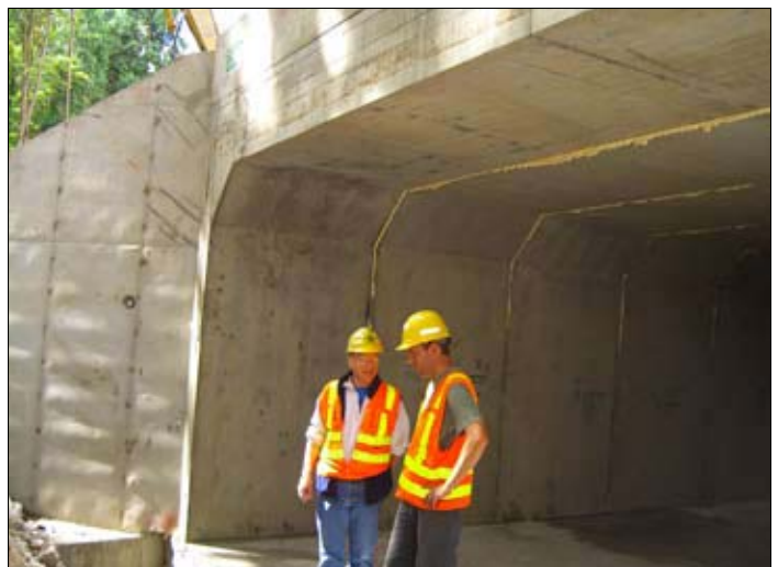
WSDOT project engineer Chris Damitio, left, and lead inspector Brian Charleston, discuss details of the culvert replacement project at Terrell Creek.
