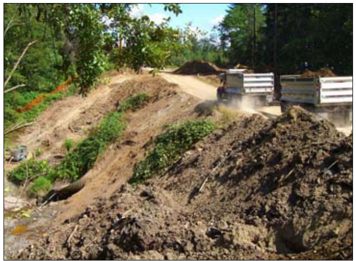
The culvert was 25 to 30 feet below the road, making it difficult to get to.
